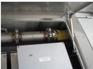
Hose connection inside lockable hose termination
